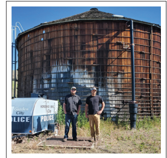
Water Operations Specialists at the Horseshoe Bend Redwood water tank during an IRWA visit.
